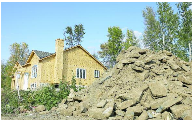
A section of property that is covered over with rocks and extra soil during home construction becomes inaccessible for use as a drainfield.
