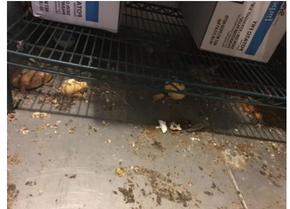
Inspection violation in a food facility
