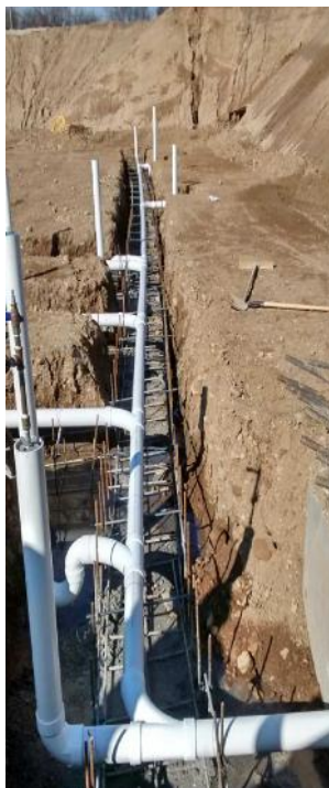
View of underground pipes at new water treatment plant in Piqua.
